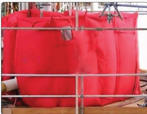
Typical welding habitat
